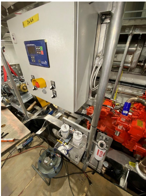
A control box for the main engine in the engine room, showing a yellow sticker with the weight of the box.
