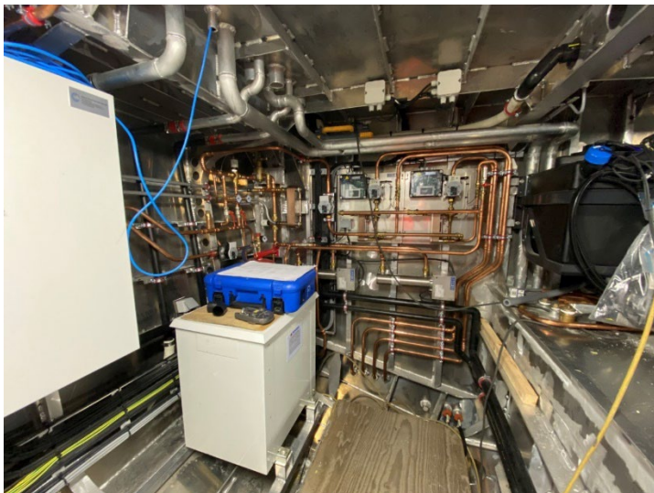
The technical space with a view of the copper pipes for the heating installation.
