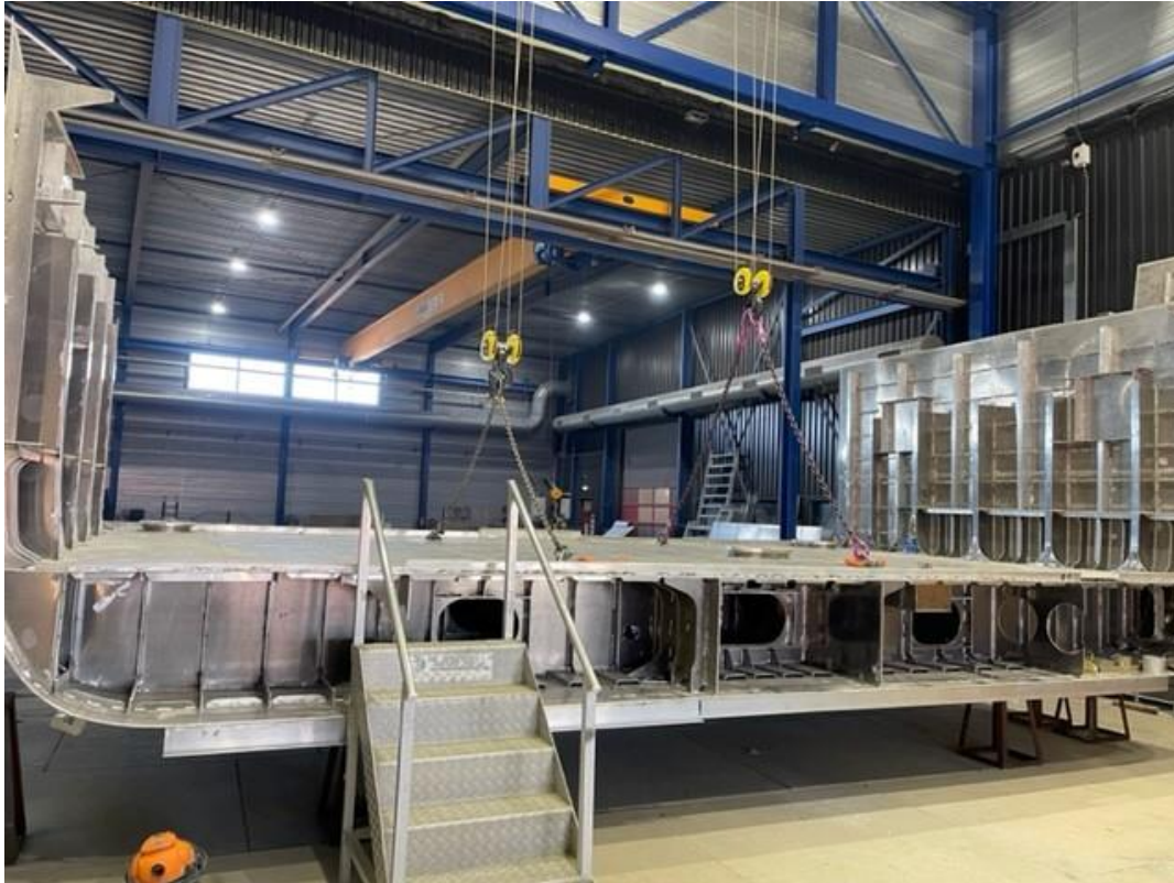
Construction of the first ring sections. Two bottom sections (330 and 340) have already been positioned for welders to join together. Work has also begun on assembling the ring by adding sections 430 and 440. ©PB
