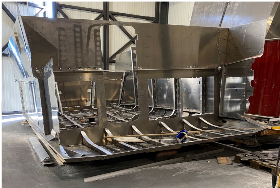
Current state of affairs late September 2021. Top: most of the hull panels have been attached. Below: the wheelhouse is ready to be attached to the hull.
