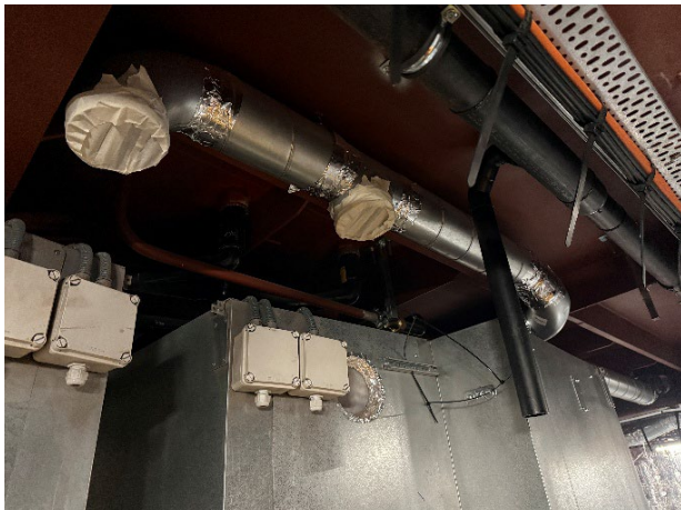
AC ducts and electrical junction boxes
