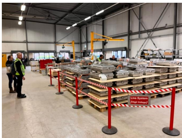
Batteries delivered to EST Floattech
