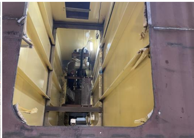
USBL trunk, with USBL pole installed
