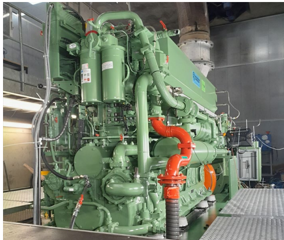
ABC 6 cylinder generator set
