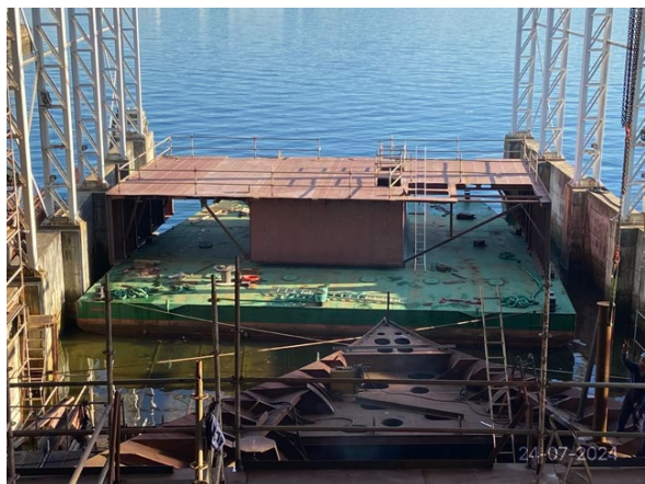
ET30 engine room with ECR ready for assembly
