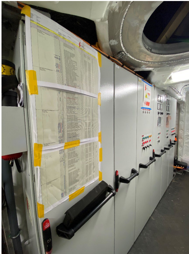
The list of alarms on a circuit breaker in the engine room switchboard locker. Each alarm is checked individually, and signed for approval.
