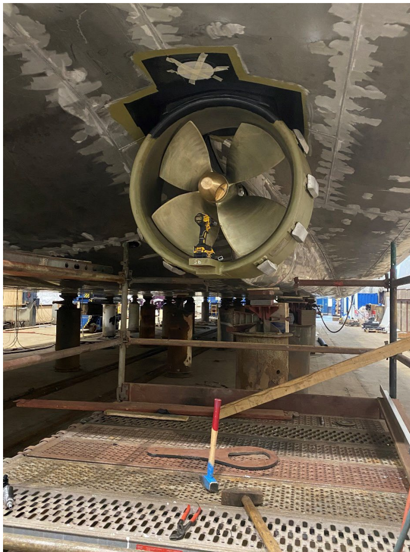
The propeller mounted in the duct on the starboard side. The rudders behind the propeller and duct housing still need to be installed. ©FH
