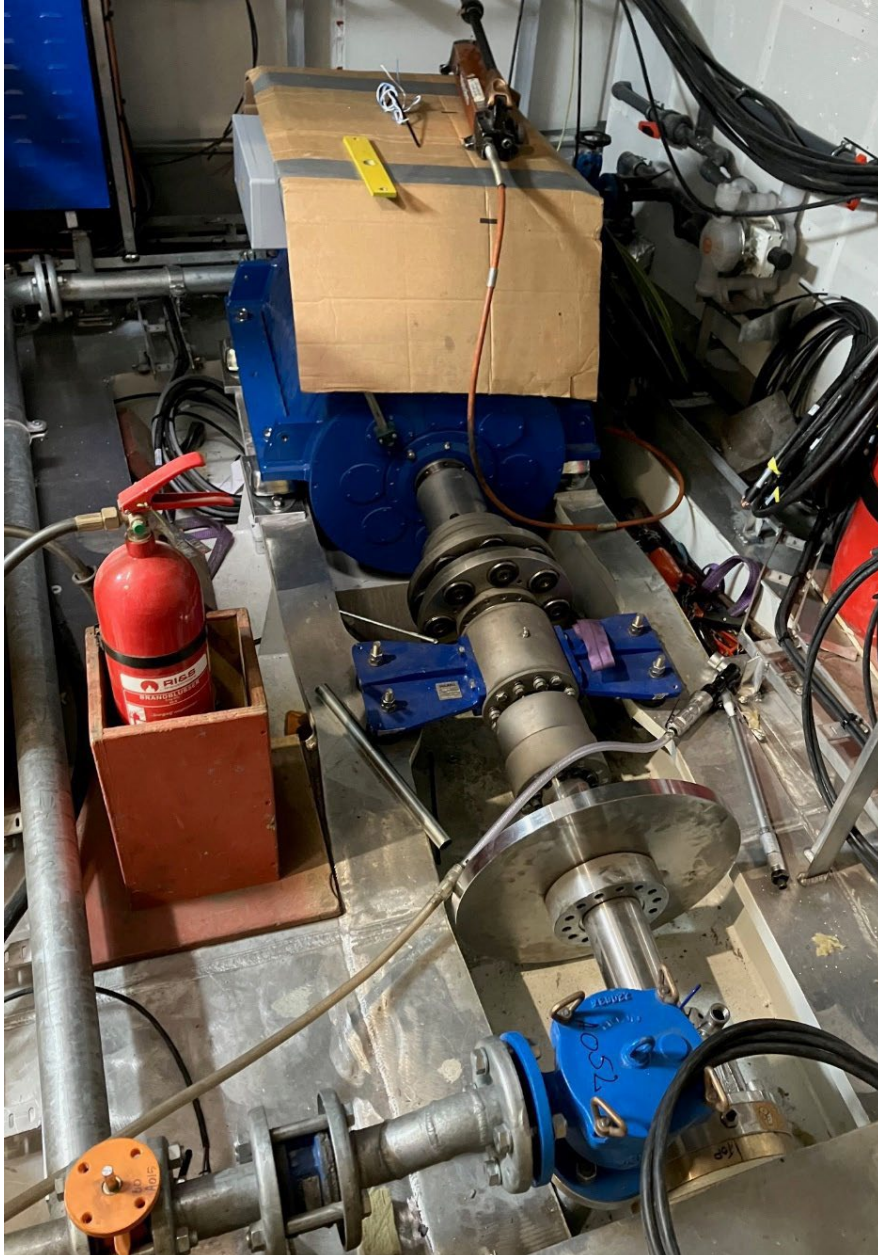
In the engine room, the propeller shafts are connected to the thrust bearing and the engine drive shaft via a flexible coupling. The propeller shaft is fitted with a brake disc that serves to block the propeller shaft, for example in the event of engine damage.
