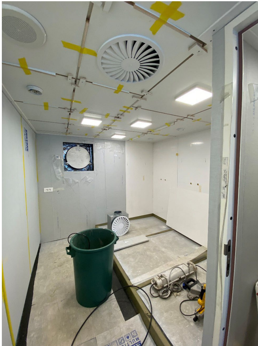
The shower cabin and head, showing the enclosed overhead.
