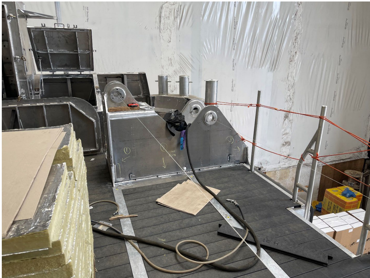
Most of the work of fitting the synthetic deck panels has already been completed. The base for the A-frame is clearly visible. ©FH
