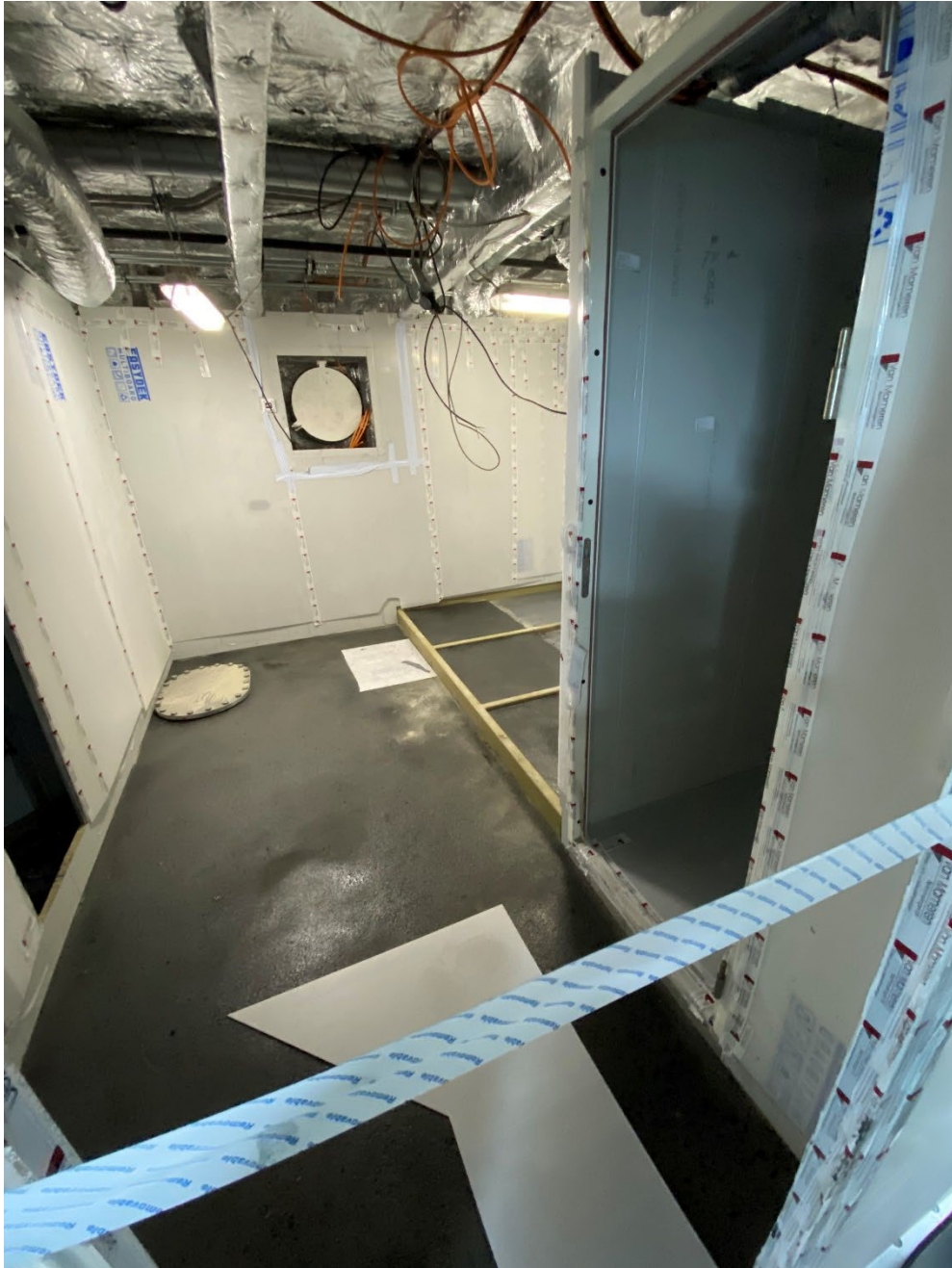
The central heads are equipped with heated decks.
