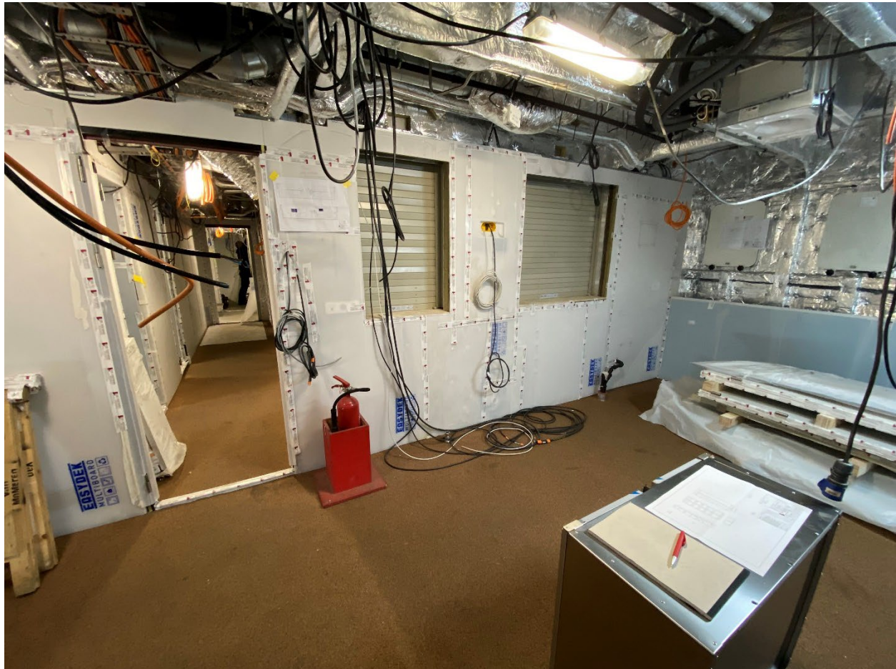
The messroom with the open overhead and bulkheads. The pass-through hatches from the galley to the messroom are also visible in the bulkhead.
