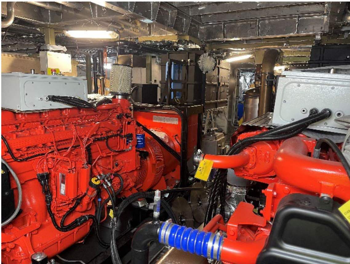
The generators in the engine room. ©FH
