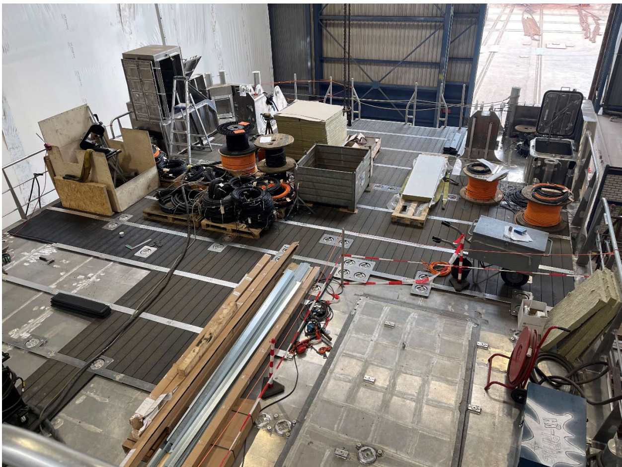
View from the bridge to the aft deck. Materials are currently being stored on the sections of the deck where the synthetic deck panels have already been installed.
