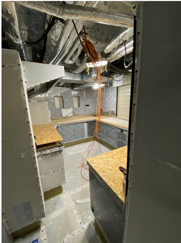
View of the galley from the passageway, showing the installed appliances.
