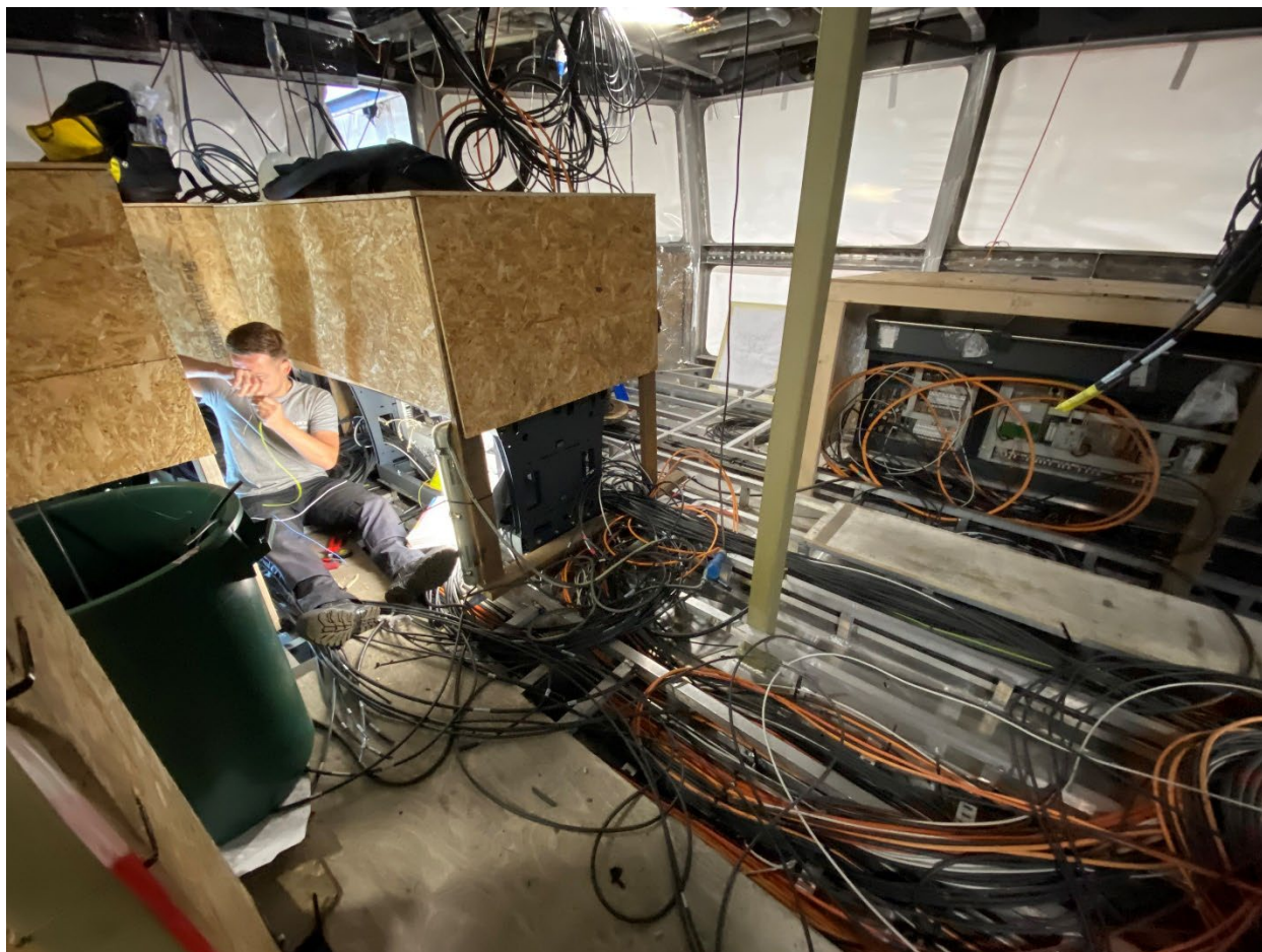
The wheelhouse, showing the housings protecting the consoles. Technicians are hard at work installing and connecting all of the cables.
