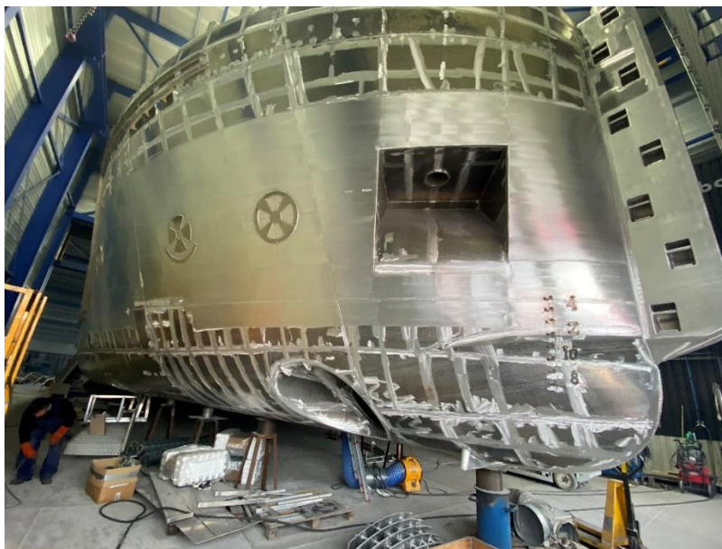
The bow nears completion, and the hull will soon be moved outside the hall. The anchor port and the bow thruster are visible.
