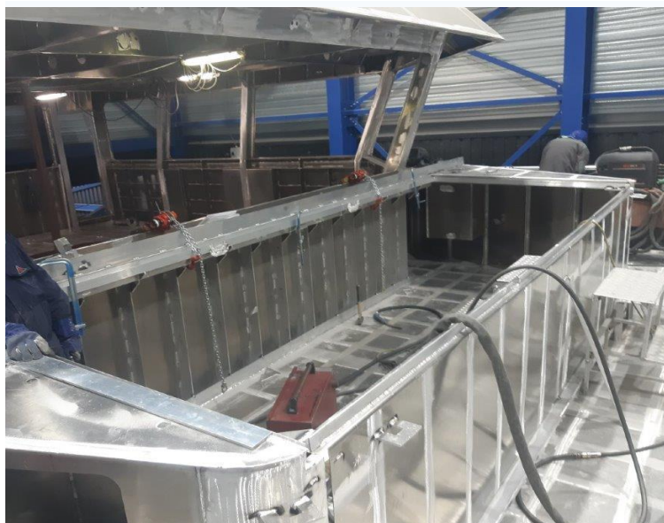
Hold for the air conditioning system.
